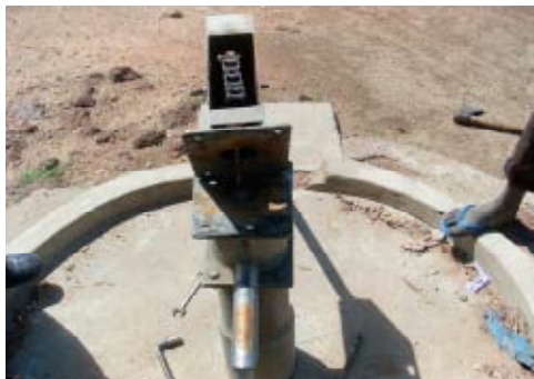
Adwir borehole before repair.
