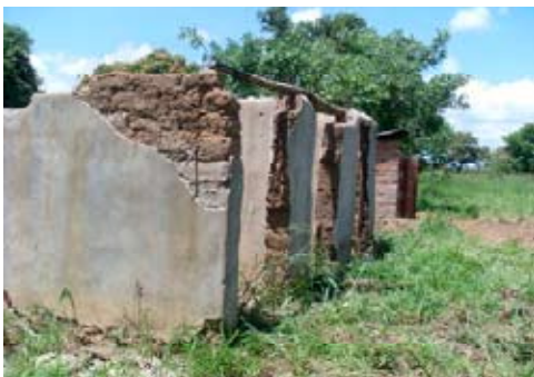
Omarari Primary School Sunken Latrines washed away by floods.
