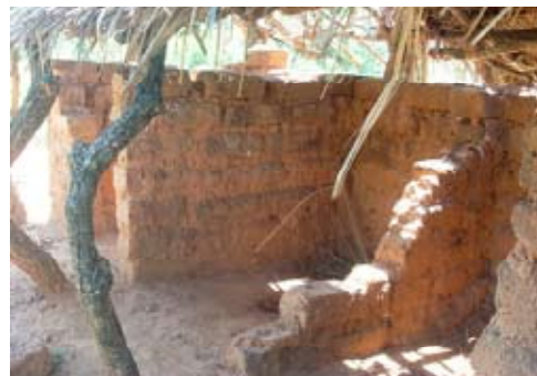
Ogongong Primary School Sunken Latrines washed away by floods.
